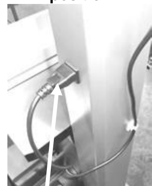
Light plugged into 110v socket
